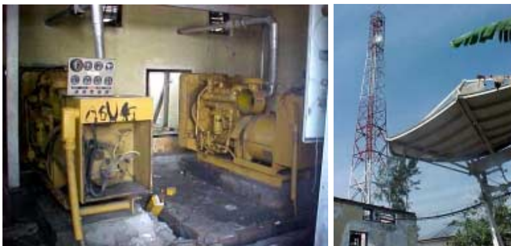
GLENO GENERATOR ROOM, RADIO TOWER
