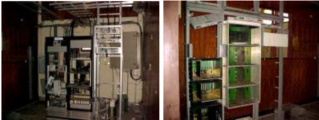
VIQUEQUE TRANSMISSION ROOM AND EXCHANGE ROOM
