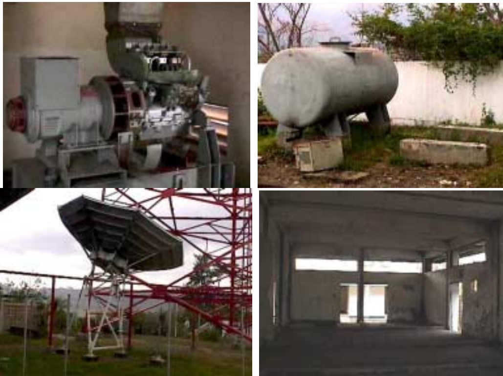
SAME GENERATOR ROOM, DIESEL TANK, SATELLITE ANTENNA AND EXCHANGE ROOM
