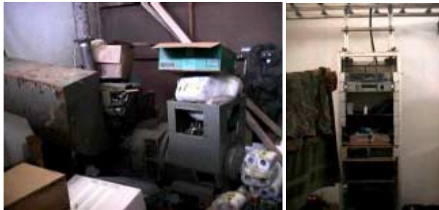
HOHONARO GENERATOR ROOM AND TRANSMISSION ROOM
